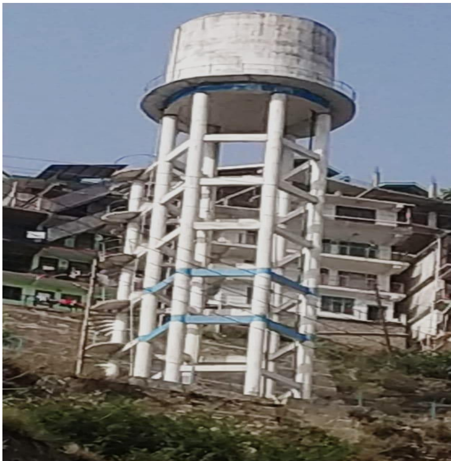
Figure 1: An overview of elevated water tank located at Jubbal, Shimla District, (HP)
