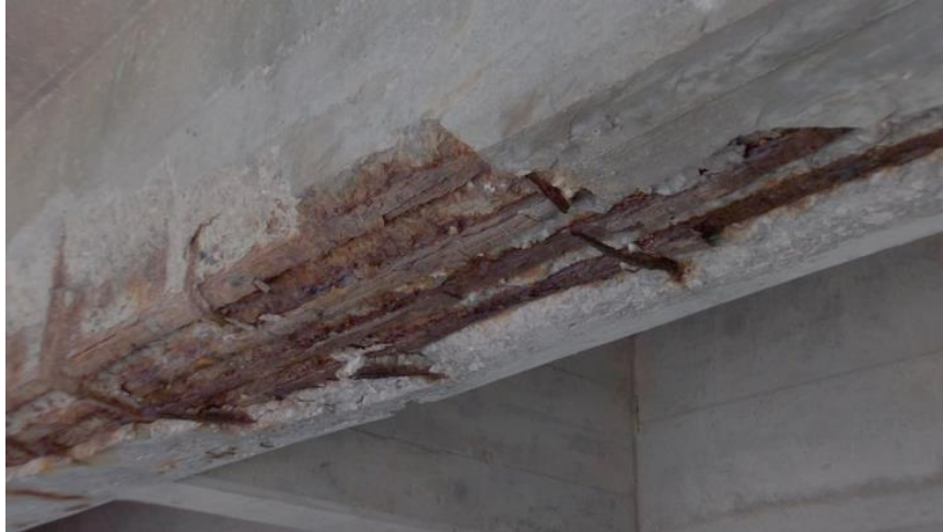
Figure 1.3 Corrosion-of-RC-structure (Source: Ju-Seong, Jung et al [10])
