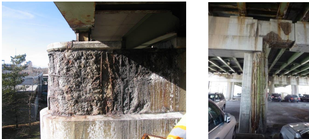
Figure 1.2 Bridges damaged corrosion due to chloride presence(Source:ENG-TIPS.com[12])
