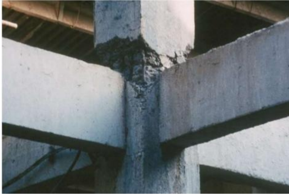
Fig. 4 :Failure of beam-column joint
