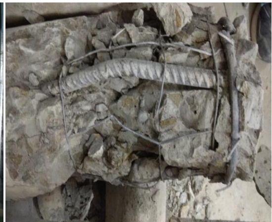
Figure 3.19 failure of column
