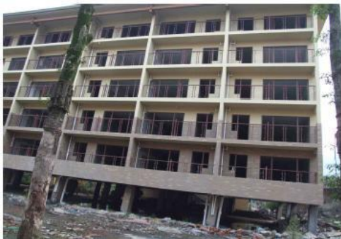
Leaned 6 story building in
