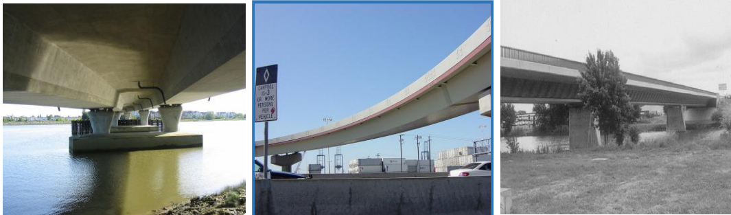
Figure 2.1: Concrete Box Bridge (Canada), San Francisco-Oakland Bay bridge (Steel Box Girder Bridge), and Cognac Bridge, France (Composite Box Girder Bridge)
