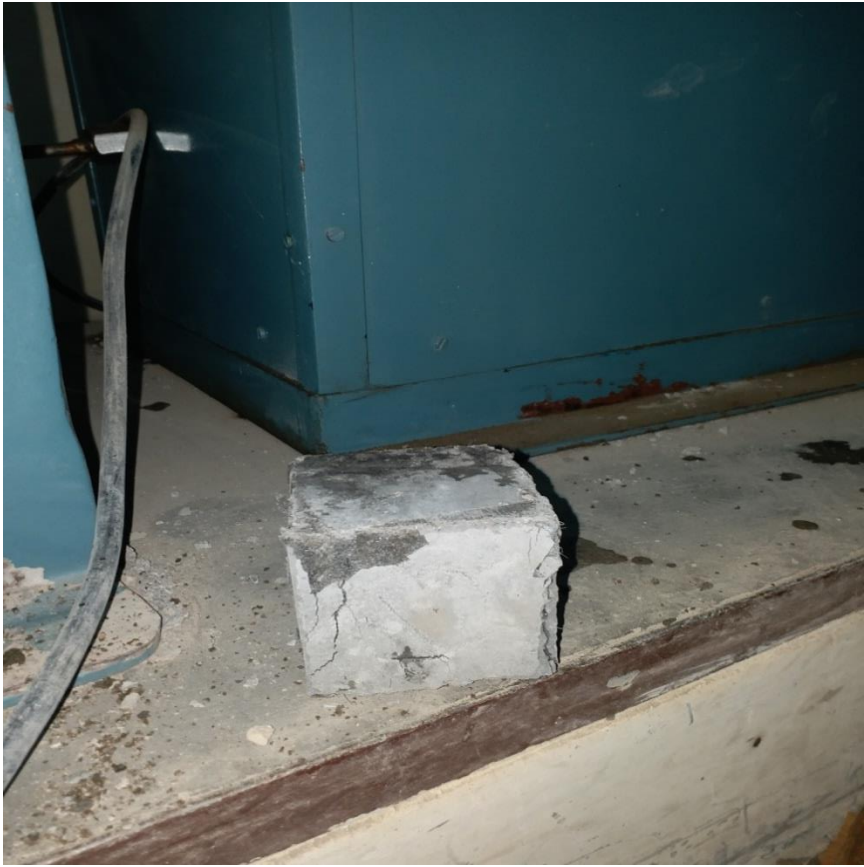
Fig.5.1. Failure of concrete
