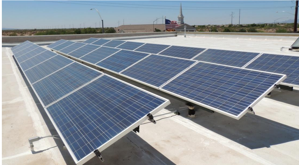
Fig – 4.12 Solar Panels
