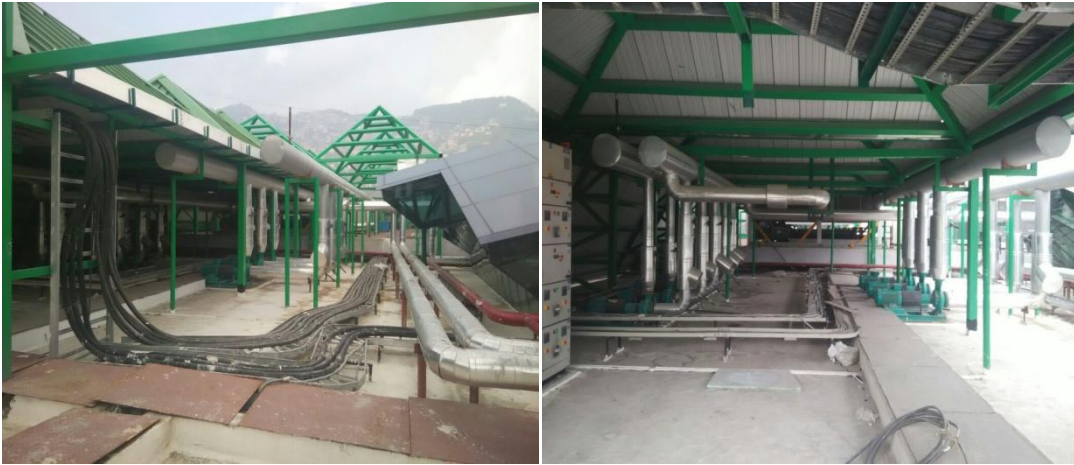
Fig – 3.5 Collector Drain Pipes in SJVNL
