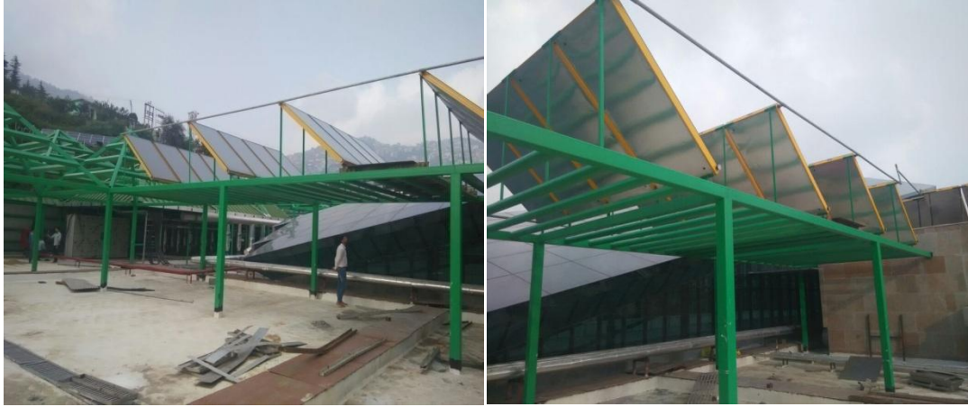
Fig – 3.4 Solar Water Heating in SJVNL
