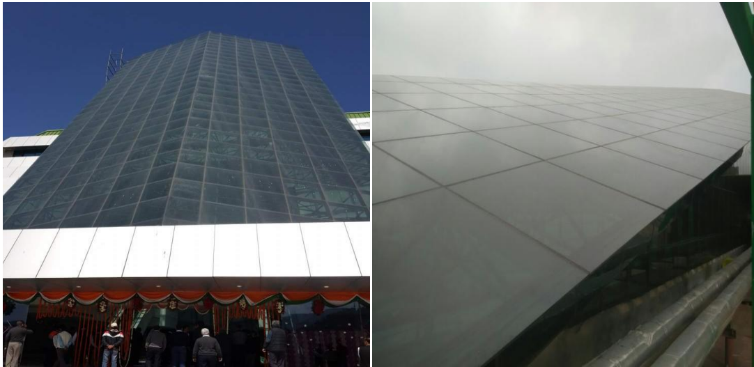
Fig – 3.3 Solar Window and Roof window used in SJVNL for Energy Efficiency
