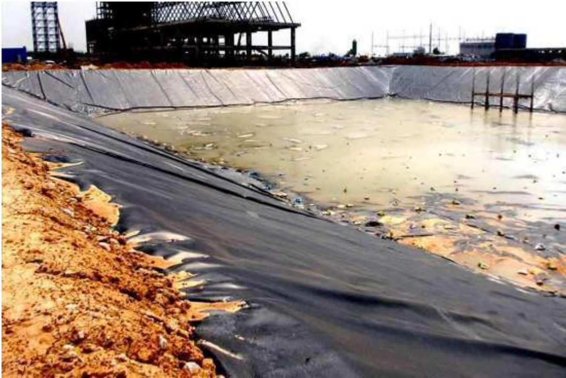
Fig. 1.10 Slope Concreting is done in order to protect geomembrane lined slope from uplift
