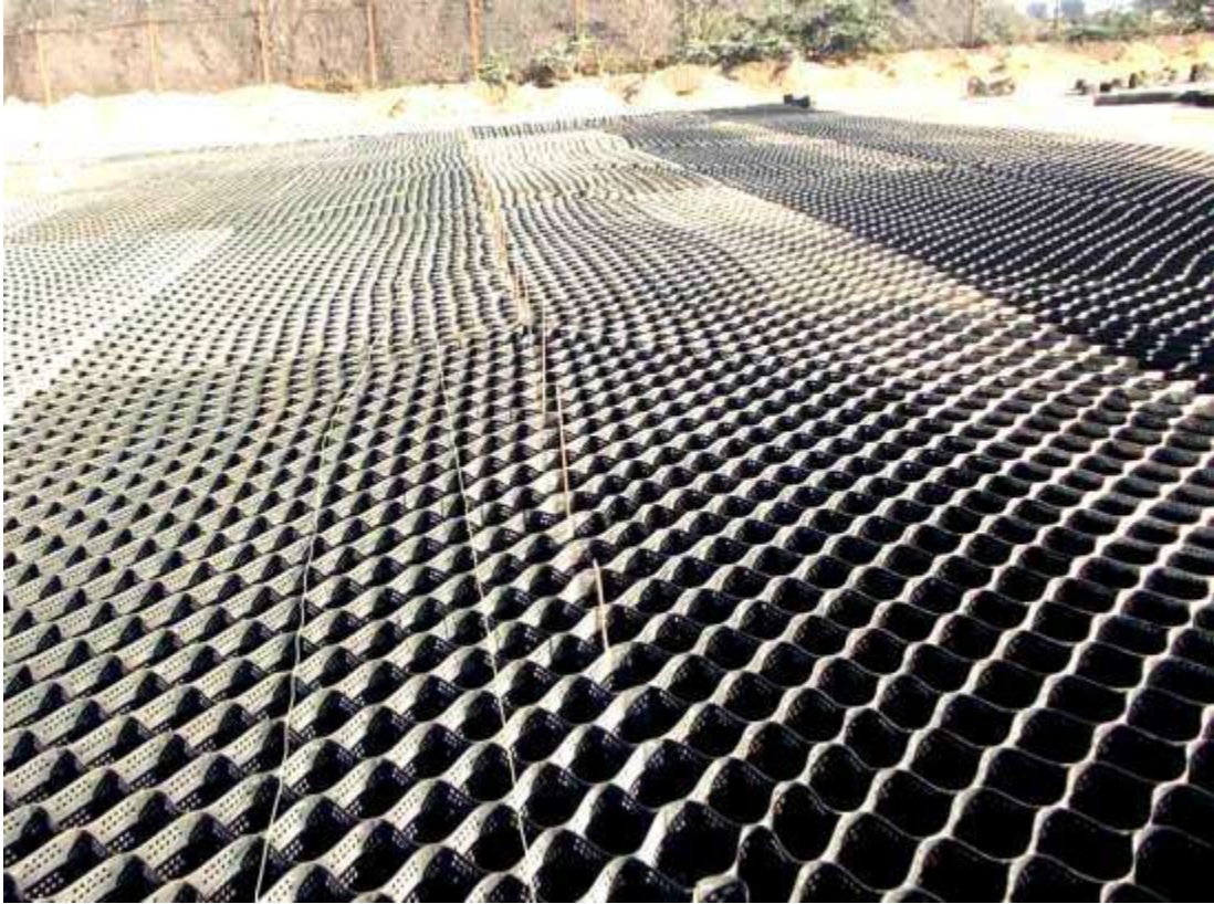
Fig. 1.8 Geocell mat spread over an area before the soil or any soil stabilized mixture is scarified over it. Thereafter the soil is tamped using vibratory roller of weight 8 to 10 tonnes and water content required. Lime stabilization is also done in order to remove excess moisture for maximum compaction of soil within geocells.
