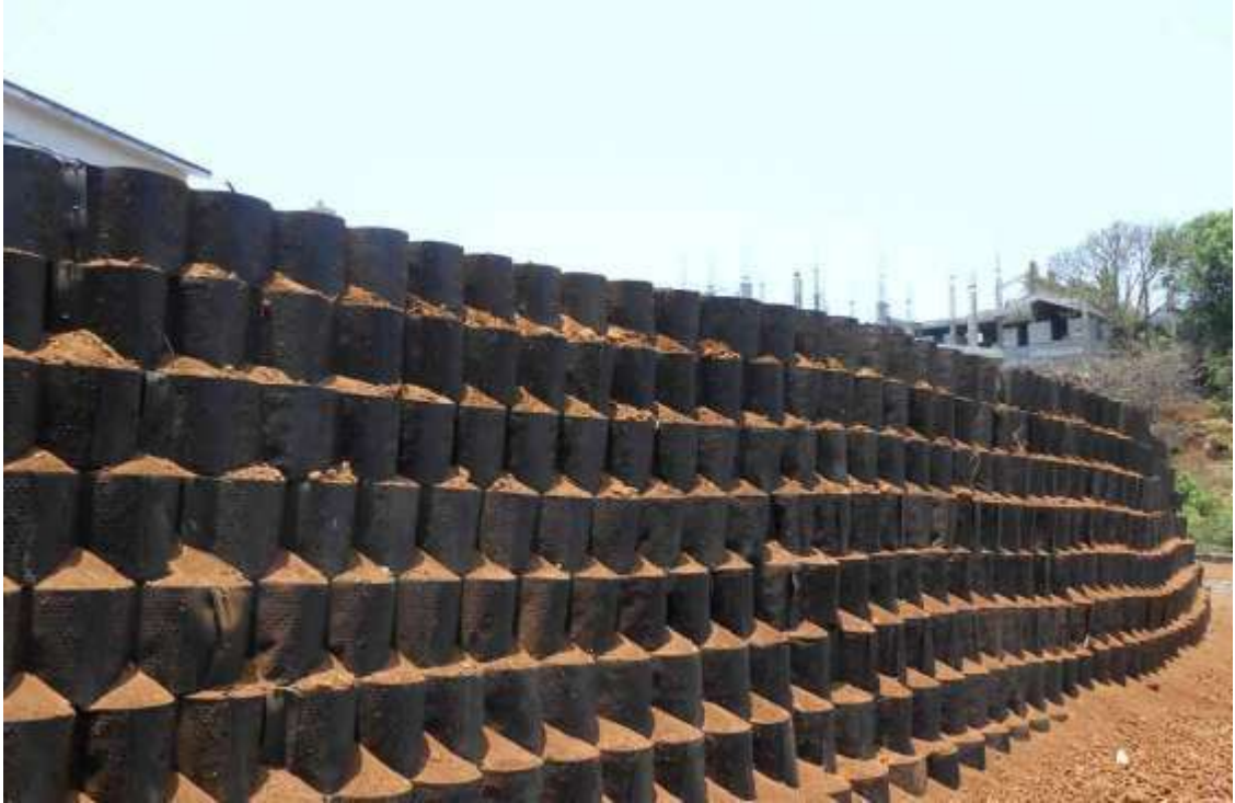
Fig. 1.9 Different layer of geocell mat are placed over each to create a mechanically stabilized retaining wall. Lime stabilization when using soil as infill and soil cement mix are generally used for placing the geocell vertically.
