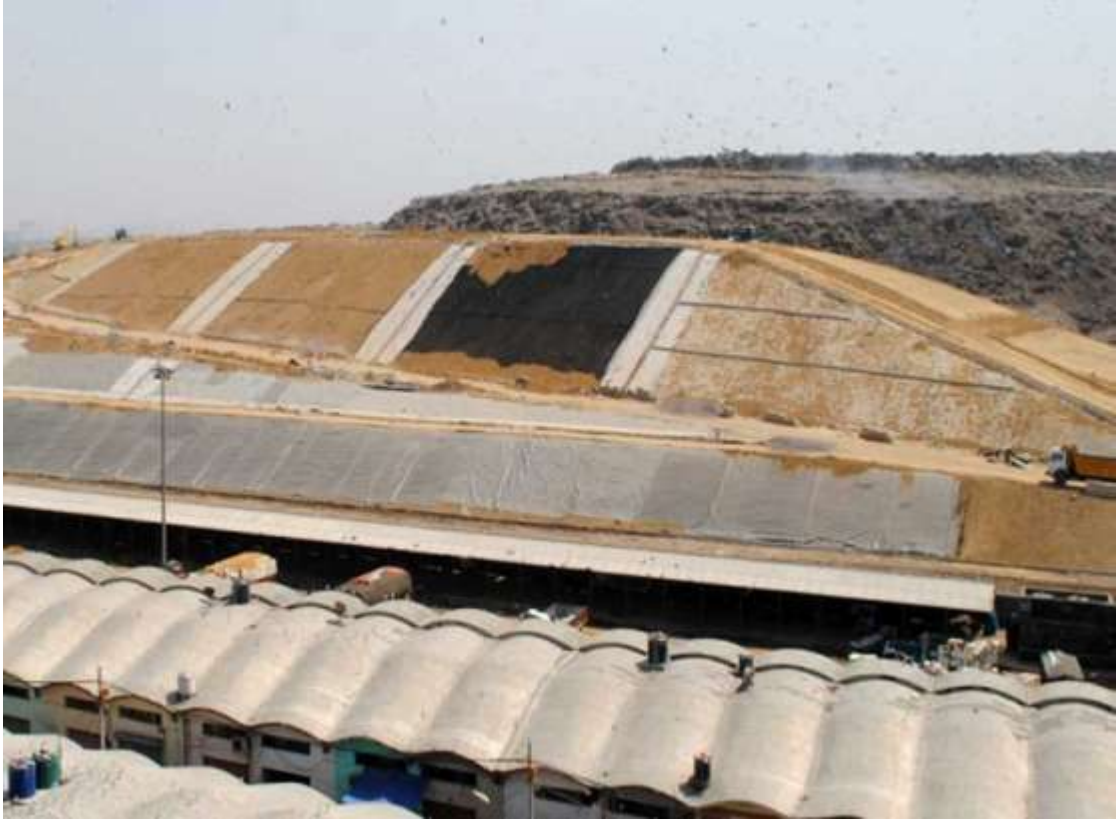
Fig. 1.7 Geocell mat laid over the slope which helps in strengthening the soil and holding the top soil layer tightly.
