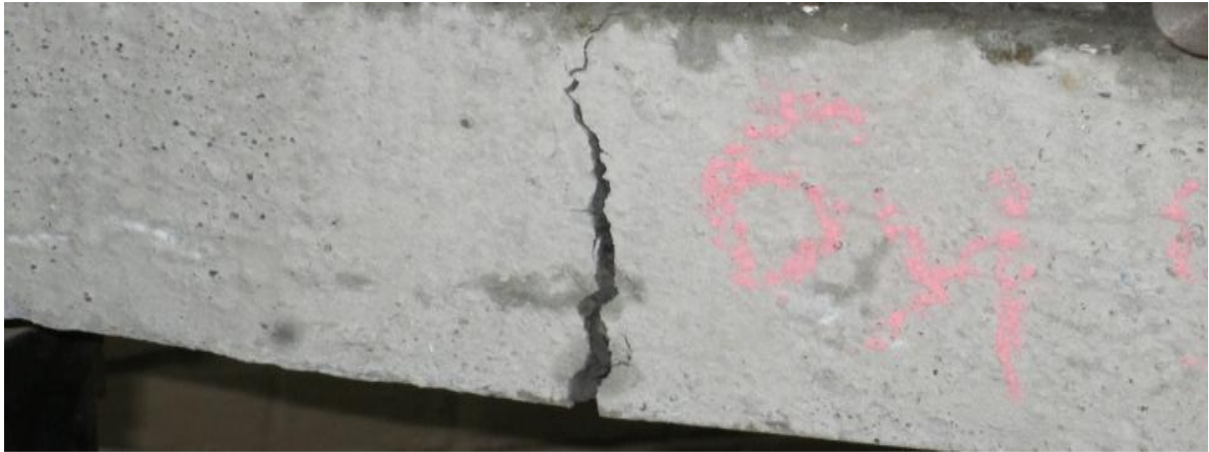
Figure 3.27 Development of Crack in Sikadur 32 gel BRC beam
