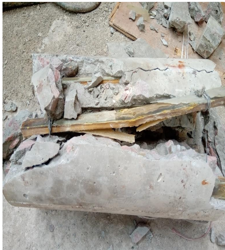
Figure 3.33 Failure of bamboo reinforcement
