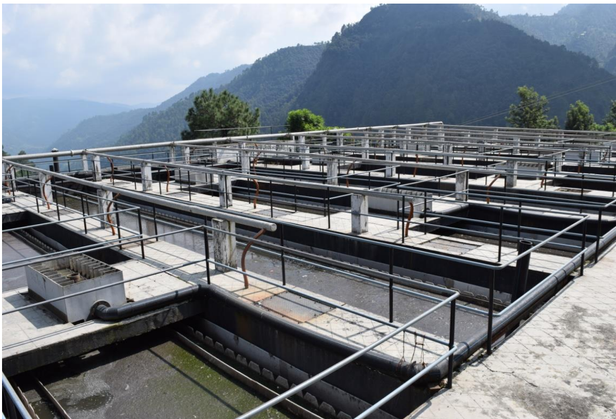
Figure 1.8: Full view of UASB reactor at Lalpani STP.
