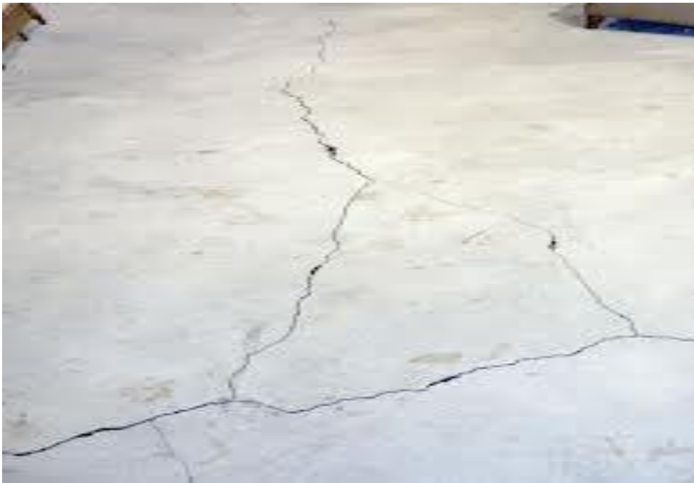
Fig(2.3) Cracking Of slabs
