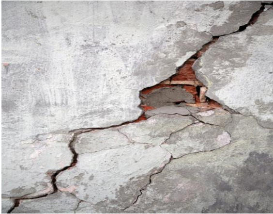
Fig(2.1) Seepage Failure
