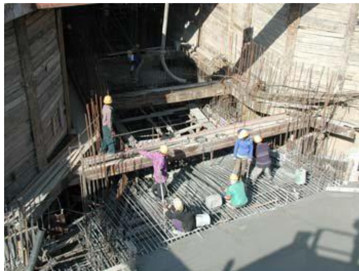
Fig. 1.5: Delhi Metro project – M35 HVFAC showed strengths close to 75 N/mm 2 after 270 days
