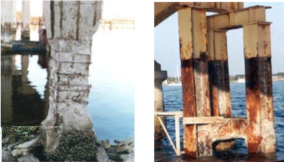
Figure 1.1 - Degradation of piles
